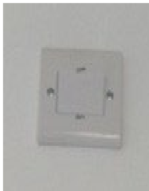
Bathroom extractor switch
